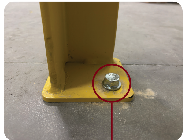
Anchor Bolts Flush with Stair
